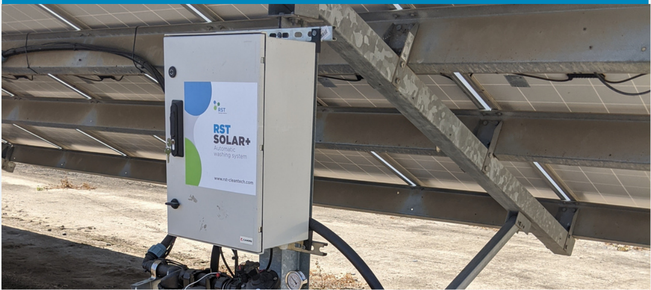
The RST control system and electrolysis system hooked up to the 1" valve and 120V outlet provided by the Leyendekkers.
