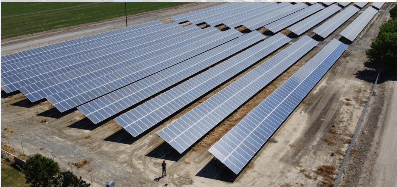
The RST system was installed on 1.5 rows of panels on the bottom right.
