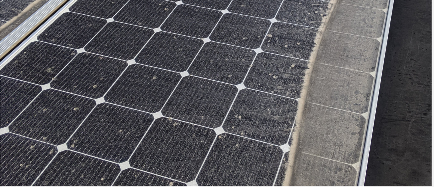
The low tilt angle on sections of the solar array contributed to soiling losses.
